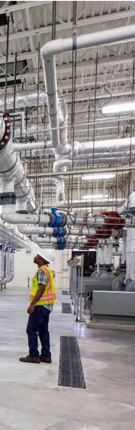
Main: Davie Water and Wastewater Treatment Plants, Davie, Florida, U.S.
